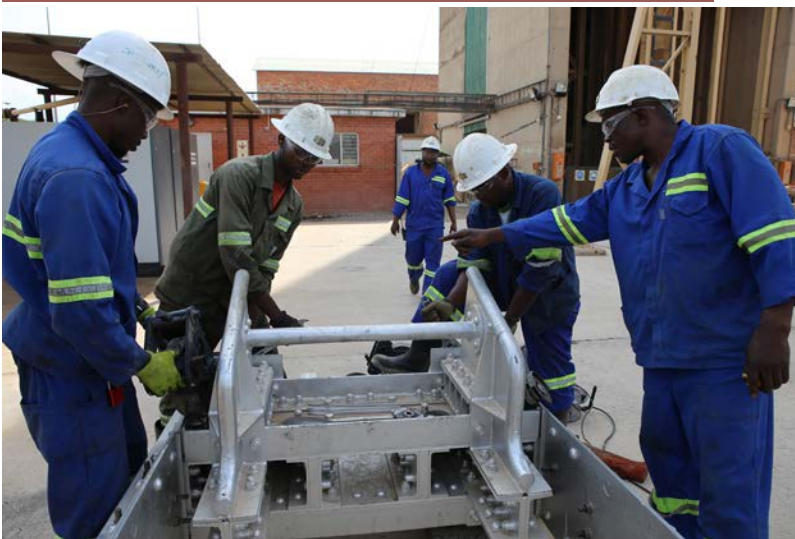
Skip assembly at the shaft (installation of cluster frames on the bridle)
