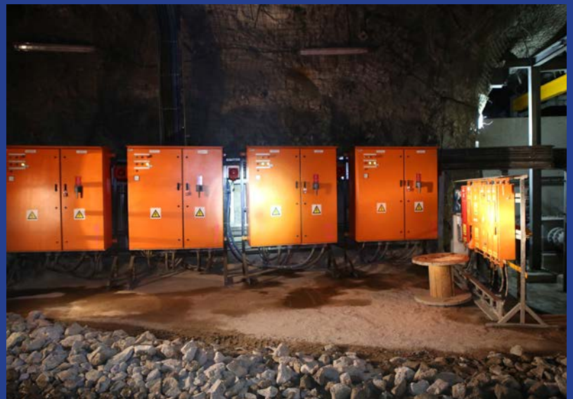
Ramp 2 – 175ml Newly commissioned Pump Chamber.
